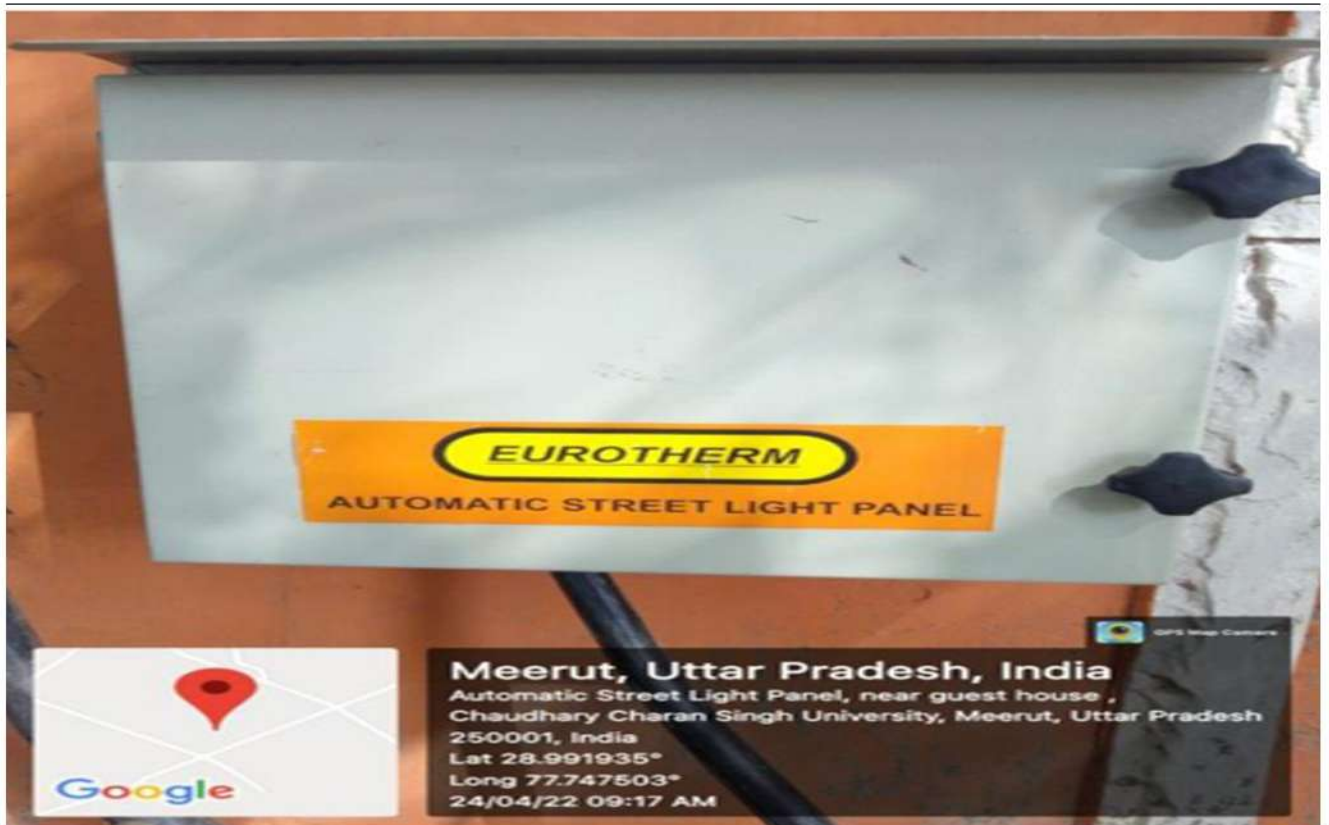
Sunlight Sensor Switch for Street Light
