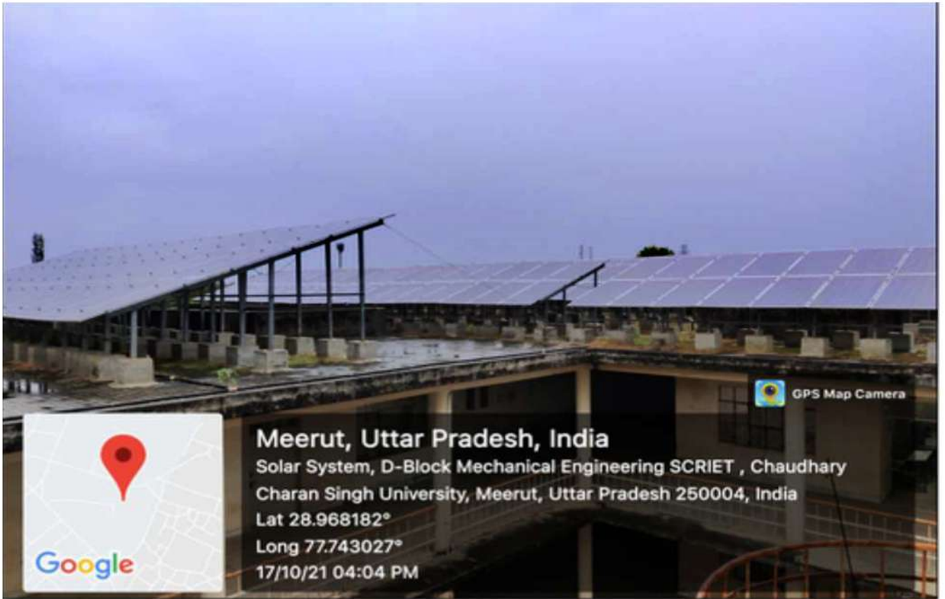
Geo-Tagged Photo - Solar Energy Panels in Engineering College
