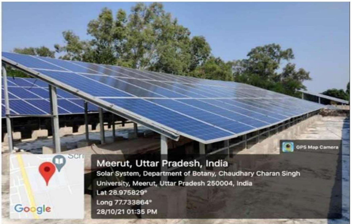
Geo-Tagged Photo - Solar Energy Panels in Applied Science Building
