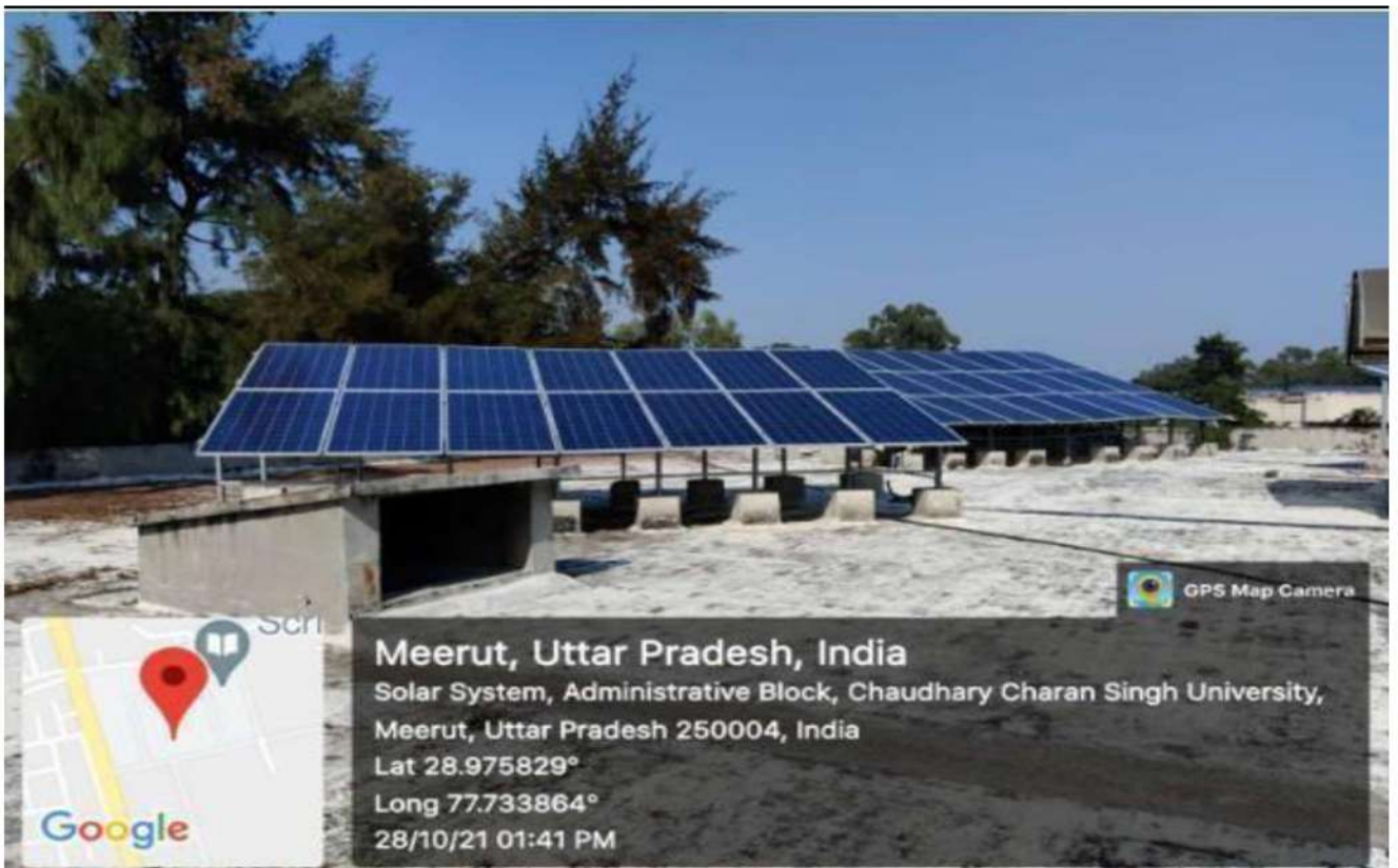
Geo- Tagged Photo - Solar Energy Panels in Administrative Building
