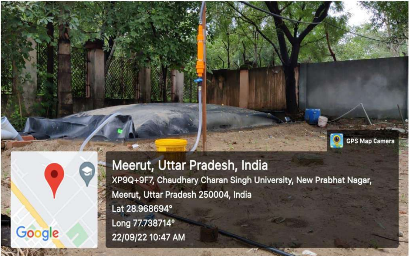
Bio Gas Plant in Dr. K.P. Hostel at University Campus
