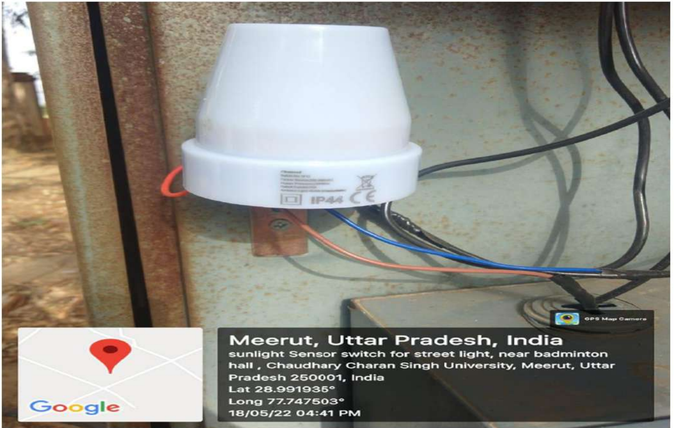
Sunlight Sensor Switch for Street Light
